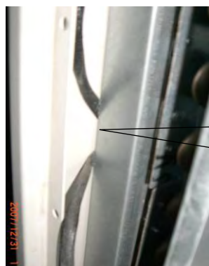
T4 sensor is worn out and connected with sheet metal
