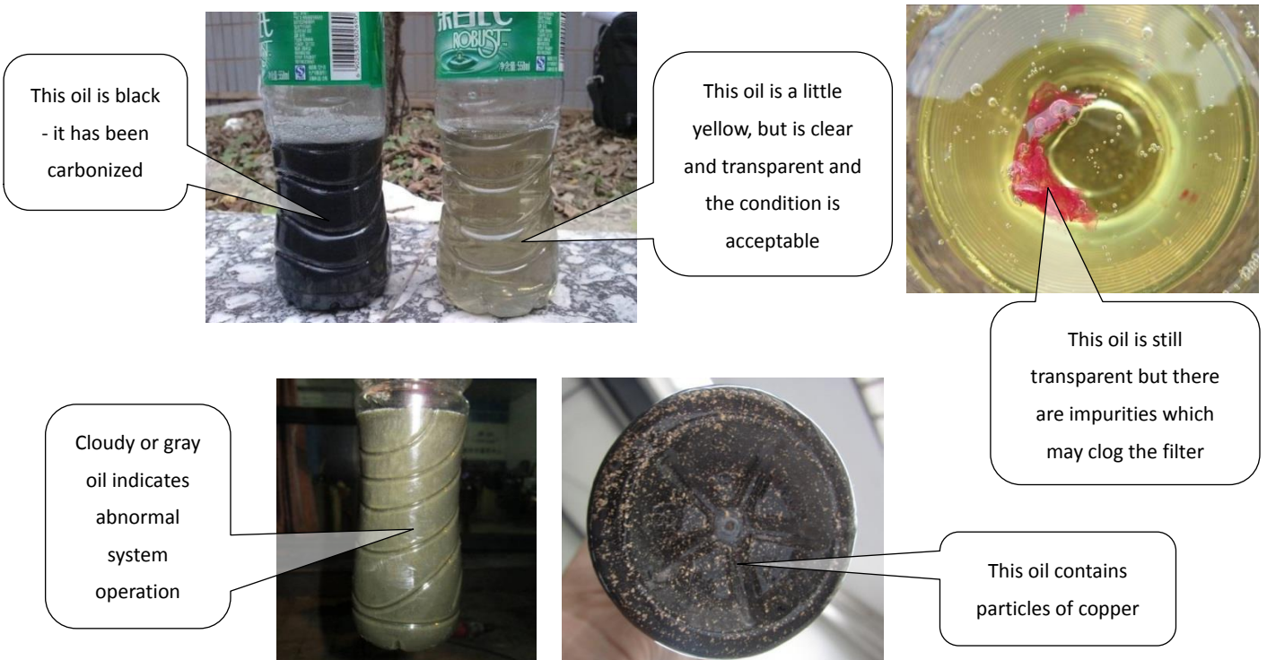
Figure 5-4.16: Inspecting compressor oil
