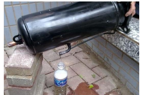
Figure 5-4.14: Draining oil from a compressor
